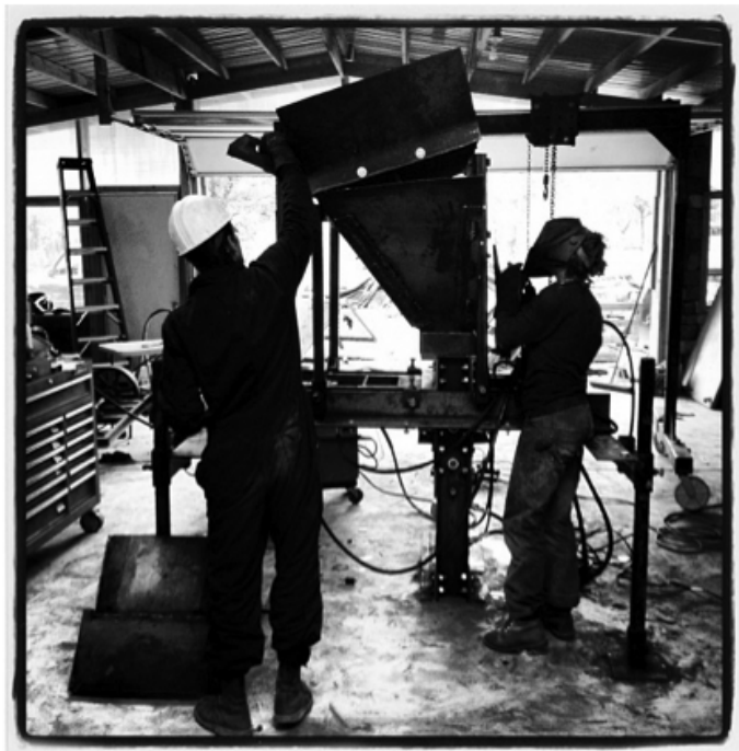
Top: Gabi, our farming manager, cutting the hopper for the compressed earth brick press
