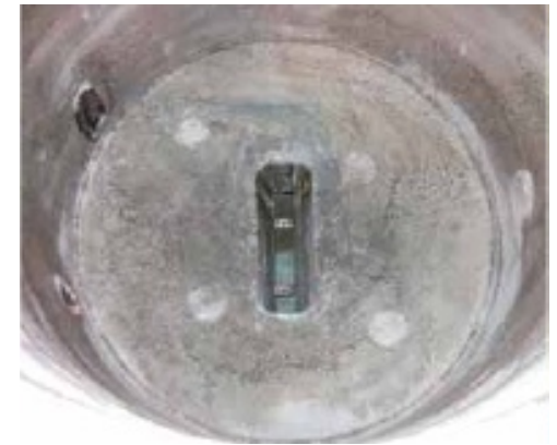
Channel inductor box lined with KELLUNDITE 857
